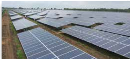
Utility Scale, Ground mounted installation, Telangana, India
