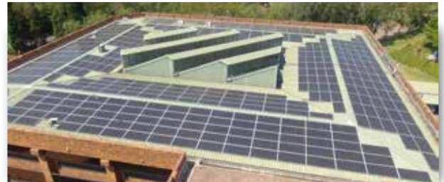
Rooftop Installation, Johannesburg, South Africa
