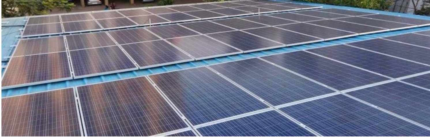
Location: Sumati Gurjar Nagar, Chembur Capacity: 50 KW
