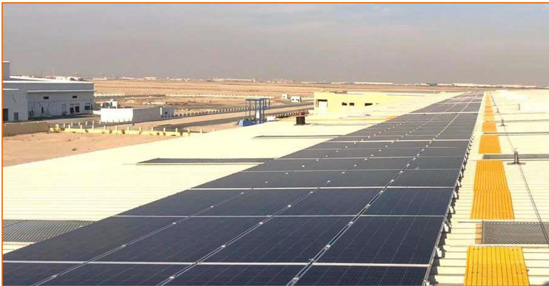
Location: DIC, Dubai Capacity: 98.3 KW
