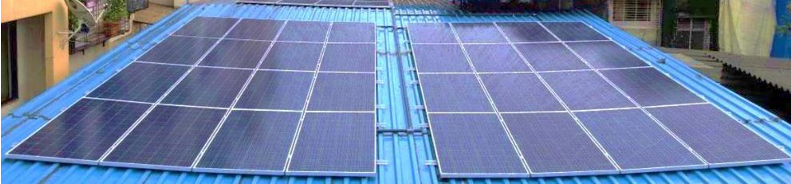
Location: Brahman Sabha, Thane Capacity: 15 KW
